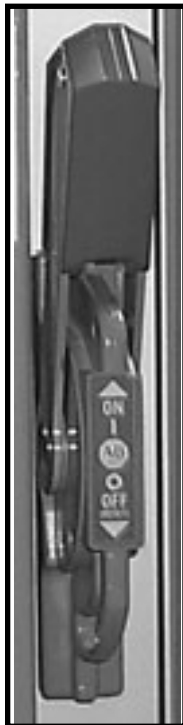
FIGURE 6-10 Main Disconnect Switch
